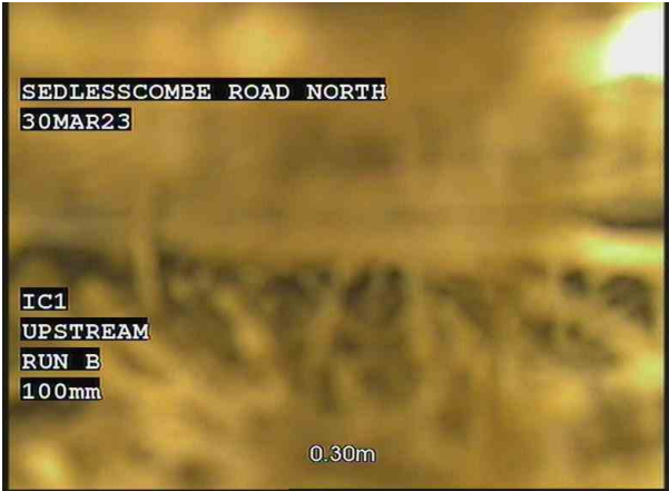
1, 00:00:11, 0.30 m Roots, mass, 20% cross-sectional area loss, start
