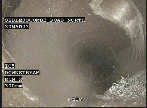
1, 00:00:32, 2.80 m Roots, mass at joint, 10% cross-sectional area loss
