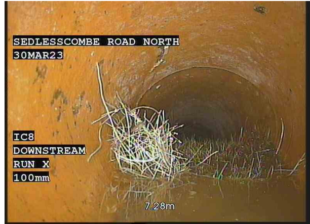
2, 00:01:15, 7.28 m Roots, mass, 55% cross-sectional area loss
