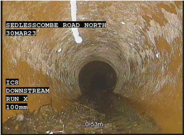
1, 00:00:09, 0.53 m Roots, mass, 20% cross-sectional area loss, start
