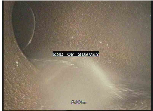
2, 00:01:50, 6.08 m Finish node, major connection without manhole, reference: RUN X, At saddle connection
