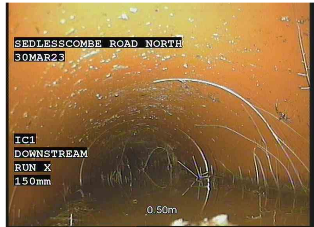
2, 00:00:18, 0.50 m Roots, mass, 30% cross-sectional area loss, start
