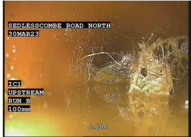
2, 00:01:09, 6.63 m Roots, mass, 30% cross-sectional area loss, start
