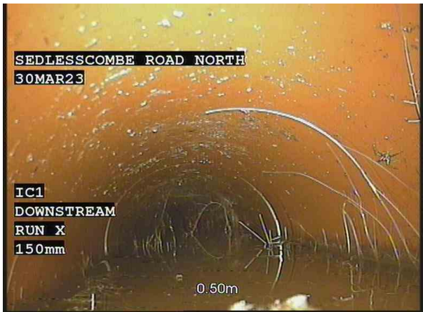
1, 00:00:12, 0.50 m Settled deposits, fine, 40% cross-sectional area loss, start
