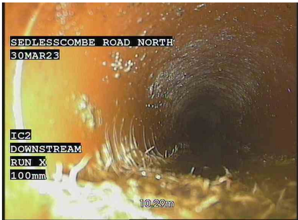
1, 00:01:02, 10.29 m Roots, mass at joint, 20% cross-sectional area loss
