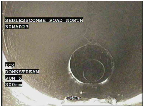
1, 00:00:10, 0.50 m Crack, longitudinal at 12 o'clock
