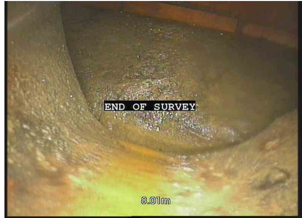
2, 00:01:06, 8.01 m Finish node, manhole, reference: 5802
