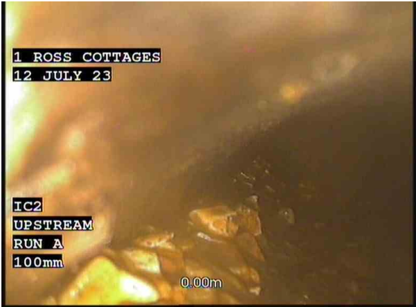
1, 00:00:01, 0.10 m Settled deposits, fine, 20% cross-sectional area loss, start, Stones
