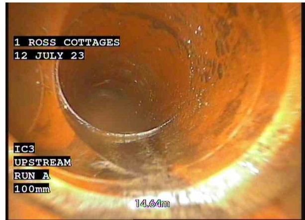
2, 00:01:23, 16.20 m Pipe material changes to polyvinyl chloride at this point
