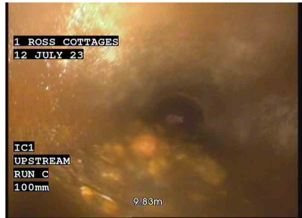
2, 00:00:40, 9.83 m Settled deposits, other, 25% cross-sectional area loss, start, Stones
