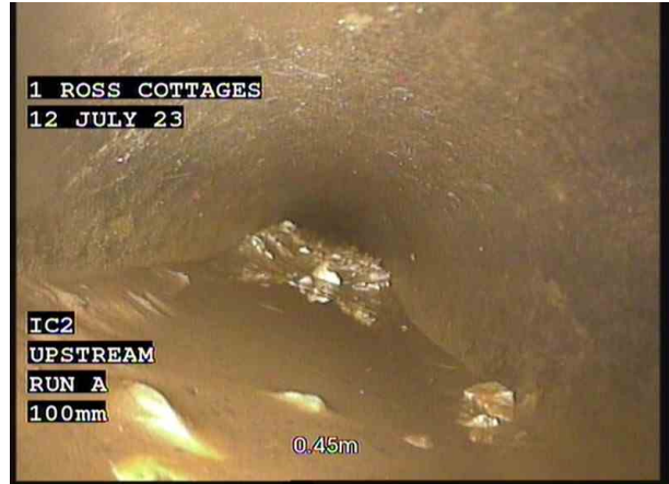
2, 00:00:29, 0.45 m Settled deposits, fine, 20% cross-sectional area loss, start
