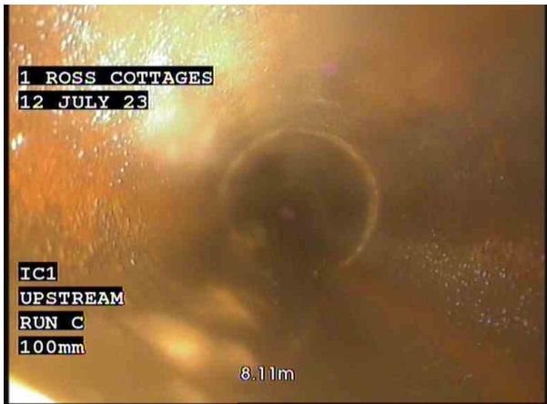
1, 00:00:33, 8.11 m Settled deposits, other, 10% cross-sectional area loss, Debris
